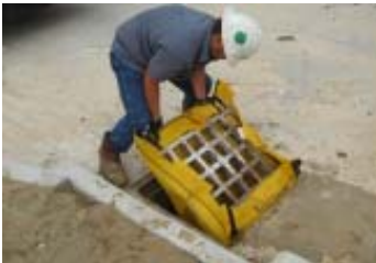
Replace Siltsack® and grate inlet into recess.
